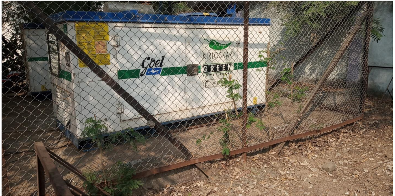
Power Generator in the Campus
