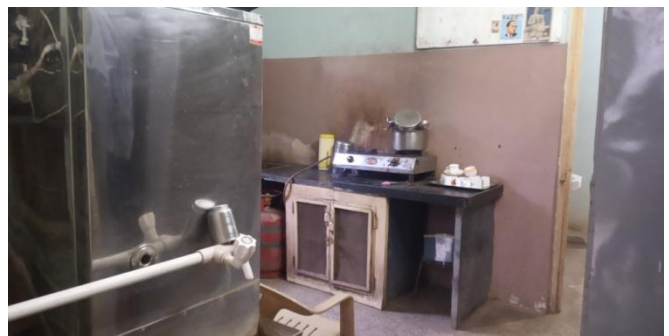
Water Filter and Chiller
